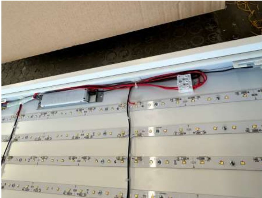
Photo 5. Electrical connections of the luminaire
